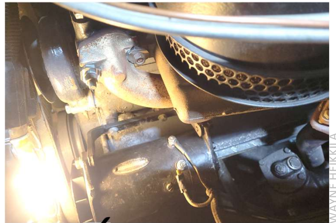
✓ Identify Coolant Leak
